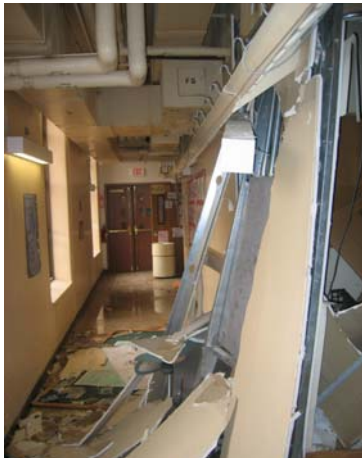
Figure 2 - Hallway Outside Laboratory Showing Explosion Damage
