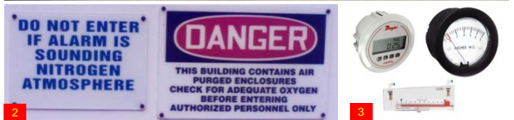
1. A pressurized and purged analyzer building (air purged with nitrogen backup) 2. Warning signs for potential nitrogen atmosphere inside enclosure 3. Examples of enclosure pressure gauges (Photos 1 and 2 courtesy of Roy E. Sanders)
