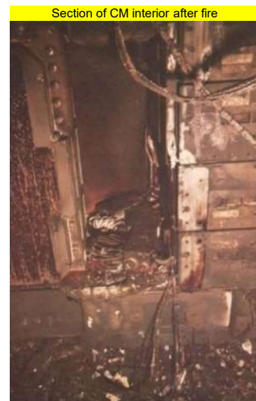
Section of CM interior after fire
